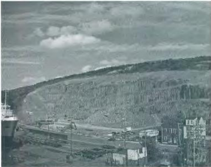
Figure 1. Southside Hill excavation. (All photographs in this article courtesy of Gerald Penney)
